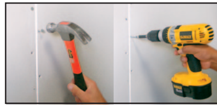
PROPERLY ATTACH PRIMED FIBERCEMENT BOARD TO STRUCTURE (LEAVE MIN. 1/8" GAP BETWEEN PANELS)
