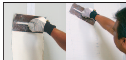
APPLY SMOOTH TO CORNERS AND JOINTS. THEN APPLY STUCCO MIX TO DESIRED TEXTURE
